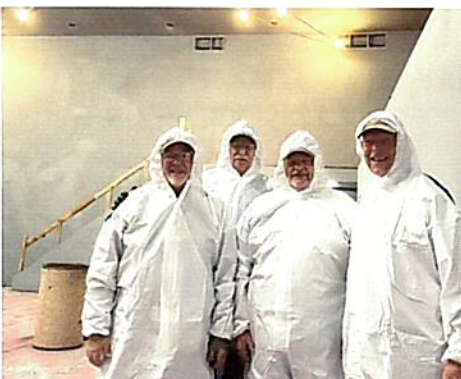
Jeff and volunteers getting ready to paint the walls and ceiling black!
